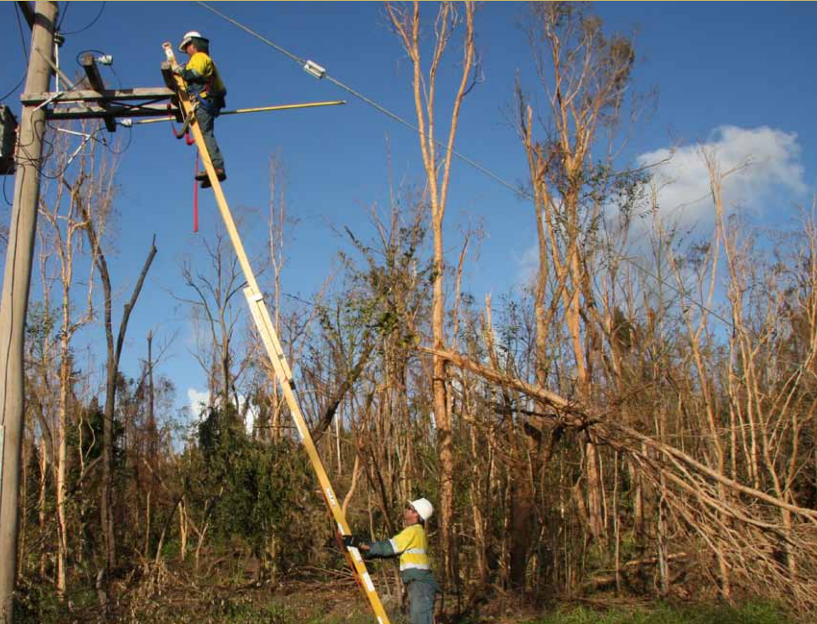
Ergon Energy workers restore power in Far North Queensland after Cyclone Yasi. © The State of Queensland.
