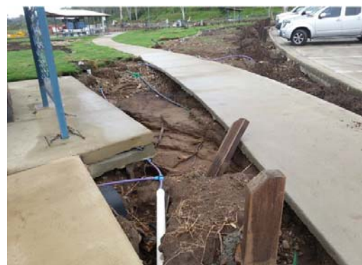
Above: damage from 2013 events to Colleges Crossing Recreation reserve (Ipswich)
