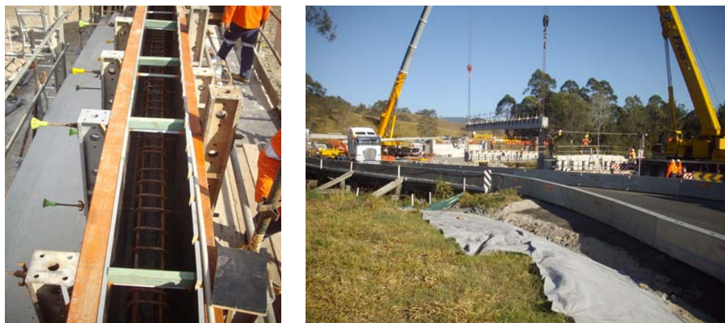
Left: Grigor Bridge ballast wall prior to pouring (left) and installing deck units in September 2013 (right).
