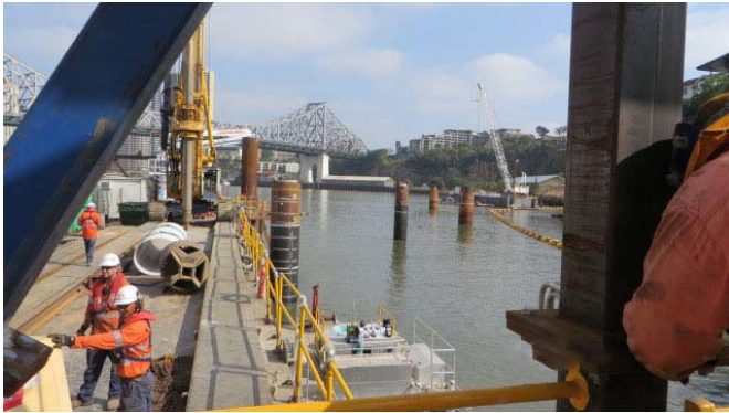
Above: looking back from the barge along the line of piles towards the Story Bridge and Howard Smith Wharves
