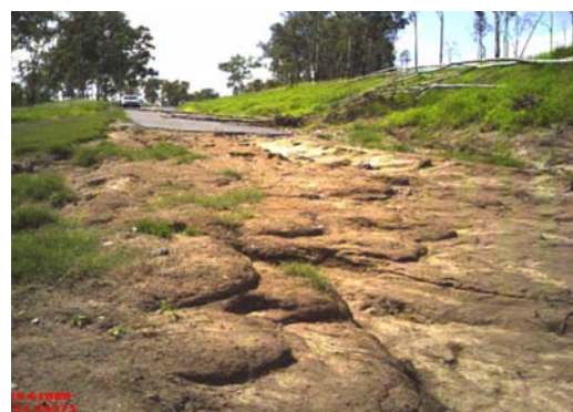
Above: 2013 event damage to Gayndah-Mundubbera Road (North Burnett)
