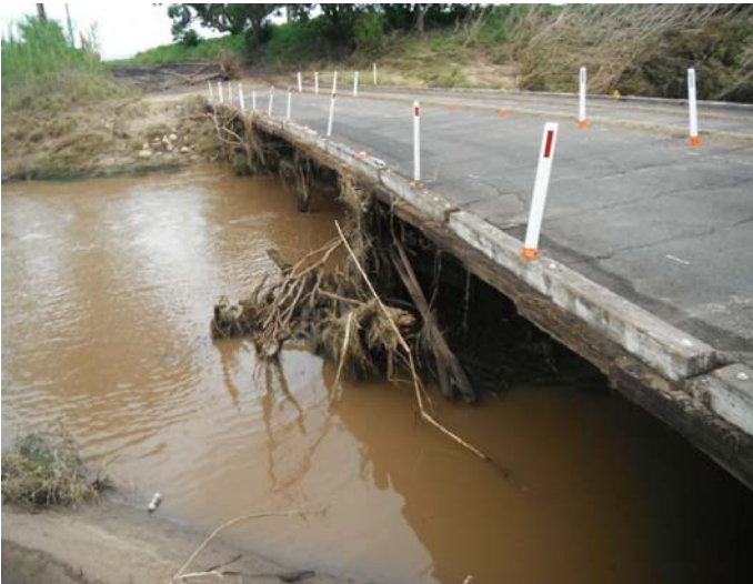
Above: Flood damaged Thistlethwaite Bridge.
