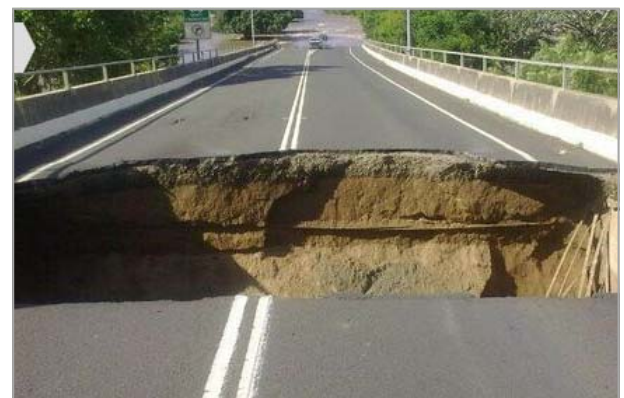
Damage to Don Tallon Bridge, Bundaberg following 2013 flood event, which was recovered within two weeks of the event, restoring a crucial cross-river link for the Bundaberg community.
